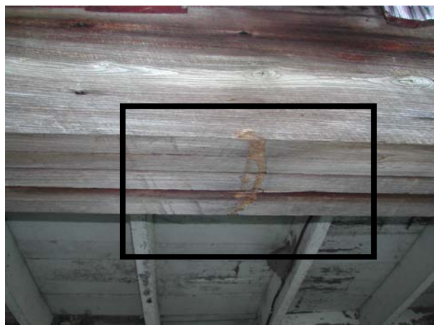
Figure 7. Mark on beam made by muffler
