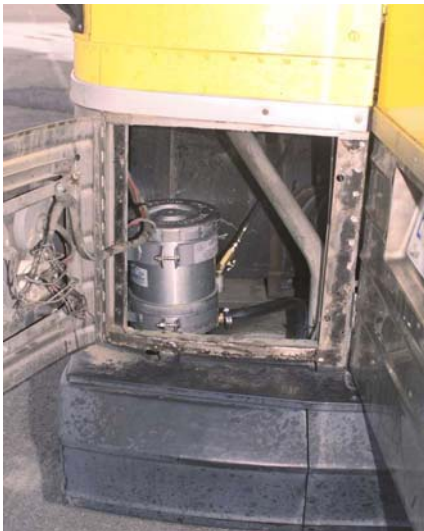
Figure 8. Close-up of filter system in rear engine compartment for a bus equipped with a Series 50 Detroit Diesel engine. The doors were installed to provide access space for the filter.
