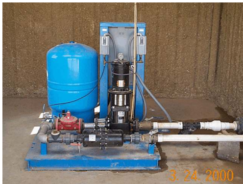
Figure 7. Pump with pressure tank and cycle-stop valve to maintain pressure on delivery line.
