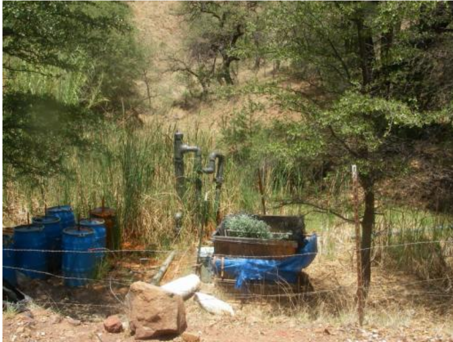
Figure 7. January Adit discharge through treatment system.
