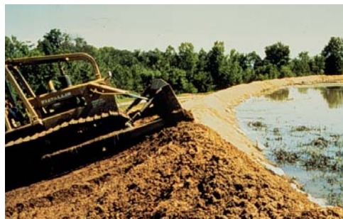
Using a bulldozer to reinforce an agricultural levee along the Upper Mississippi River near Quincy, IL during the 1993 flood.
