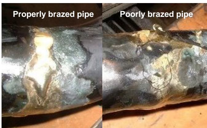
Poorly brazed pipes led to the electrical shortage that led to the loss of the USS THRESHER.
