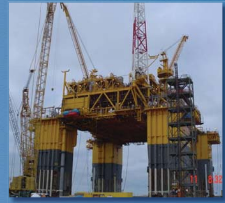
Production begins on the Independence Hub, the deepest production platform ever installed and the world's largest offshore natural gas processing facility
