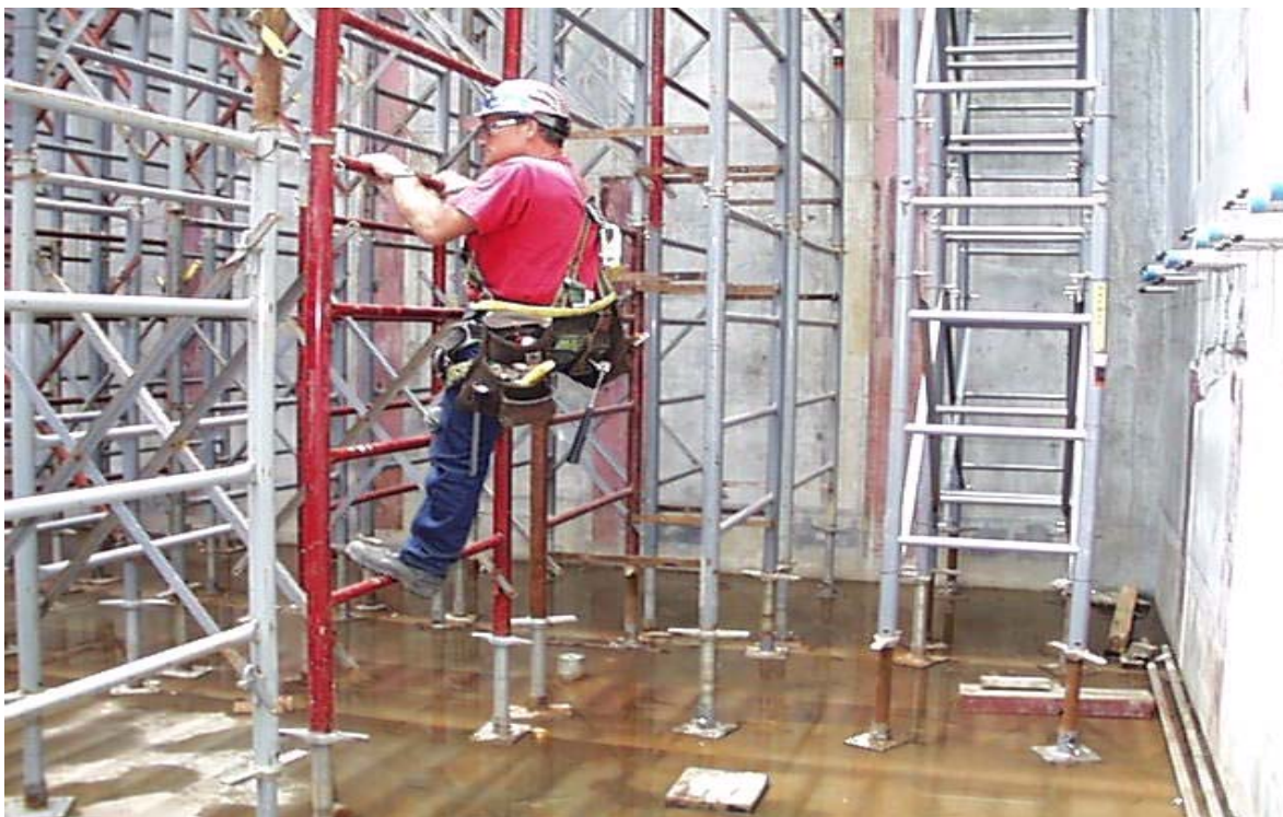
Figure 7 - Re-enactment of C1's position on shoring at time of fall
