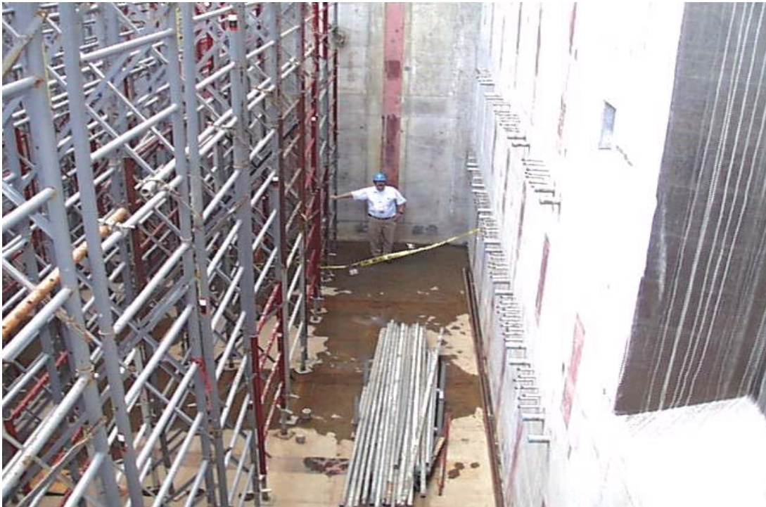
Figure 3 – Accident site (single person stairway out of view in foreground)
