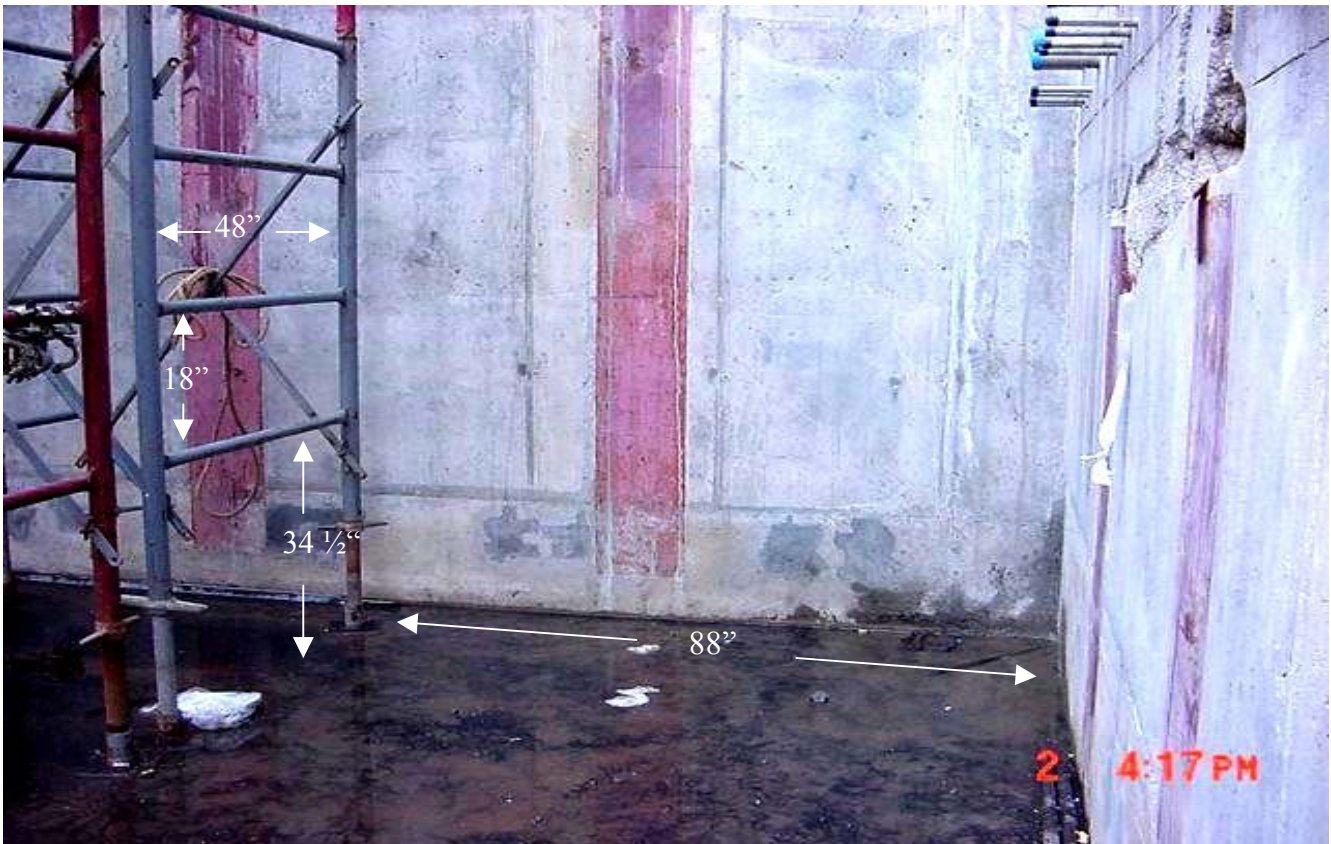
Figure 6 - Actual Accident Scene
