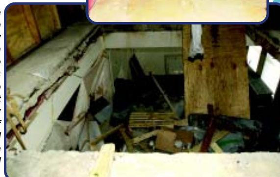
Demolition of the floor for the installation of new stair tower. Demolition is needed to upgrade and improve the MIB's infrastructure to conform to current health and safety standards. Portions of the fire protection and alarm systems will be upgraded and portions replaced.
