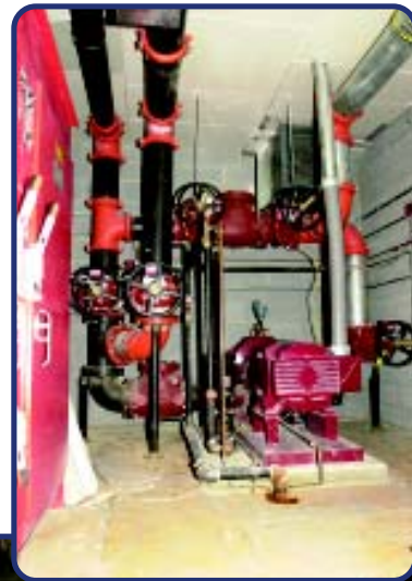
In 2003, a new fire pump was installed in the basement mechanical room.
