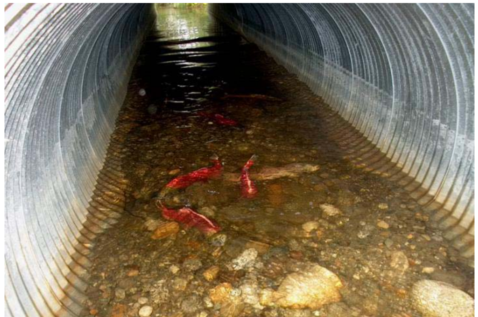
Sockeye salmon spawn in culvert with bottom designed to replicate the natural stream bed. Photo: Neil Stichert.
