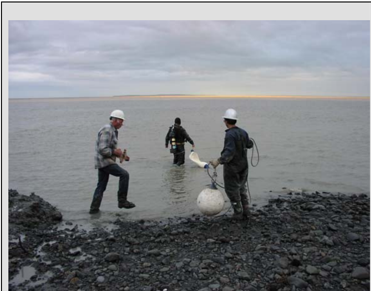
A diver wades into the Nushagak River to plug the end of the sewer outfall.
