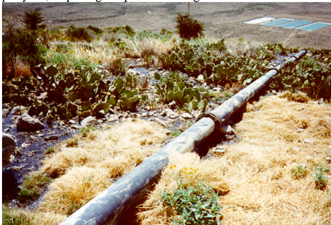
Main sewer line leak discovered in early June, 1998. Sewage is flowing from left of photo. Note sewage lagoons in the background. (NPS Photo by Dale Pate)
