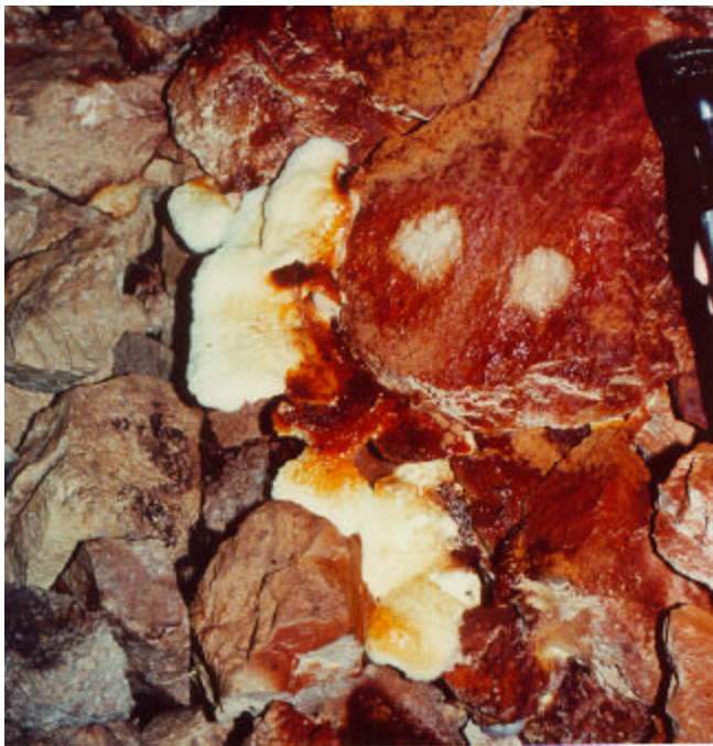
Suspected sewer leak in the Main Corridor. The large white objects are shelf fungi and the red discoloration appears to be iron that has been deposited from ceiling drips. High fecal bacteria counts were found in the dripping waters. (NPS Photo by Dale Pate)
