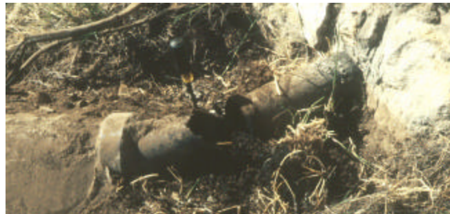
A missing section of sewer line outside Building 7. (NPS Photo taken in March 1995 by Dale Pate)
