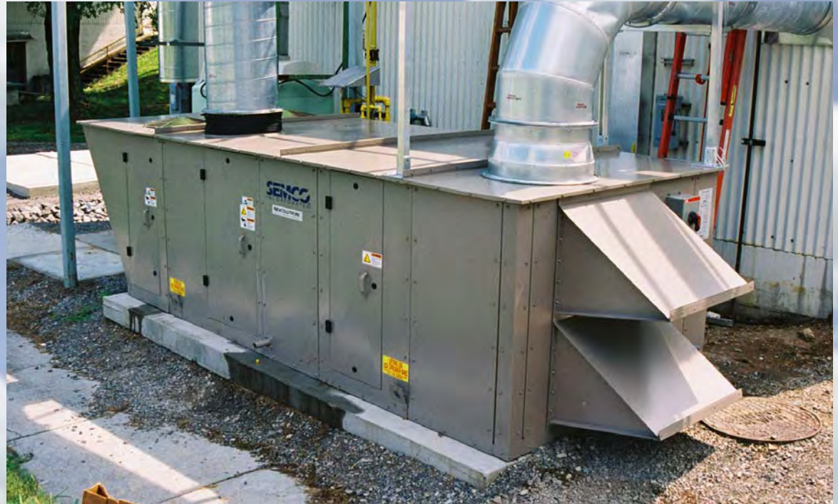
REV 2250 installed at the Oak Ridge CHP Lab
