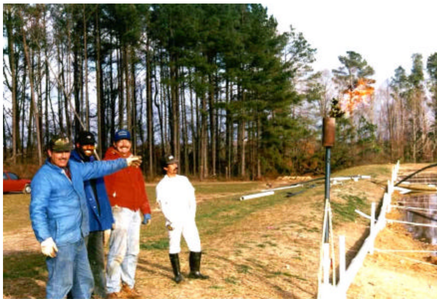
Odors go up in smoke. Installation Crew at first gas flare lighting, North Carolina.
