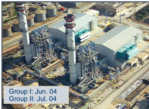
CCGT NGS - 800 MW 1
