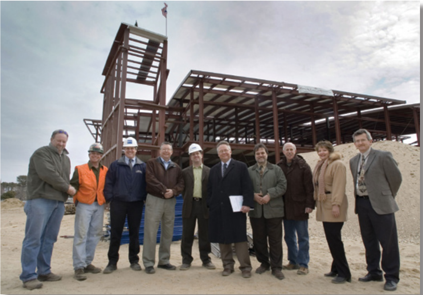
Construction on the Lab's 94,500-square-foot Center for Functional Nanomaterials started on September 13, 2005, and steel erection began on January 21, 2006. Gathered in front of the steel framework when construction workers bolted in the final steel beam for the facility, the occasion known as "topping out," are Brookhaven employees; representatives from the U.S. Department of Energy, which funded the project; general contractor E.W. Howell, Inc.; and architectural engineering firm HDR Architecture, Inc.
