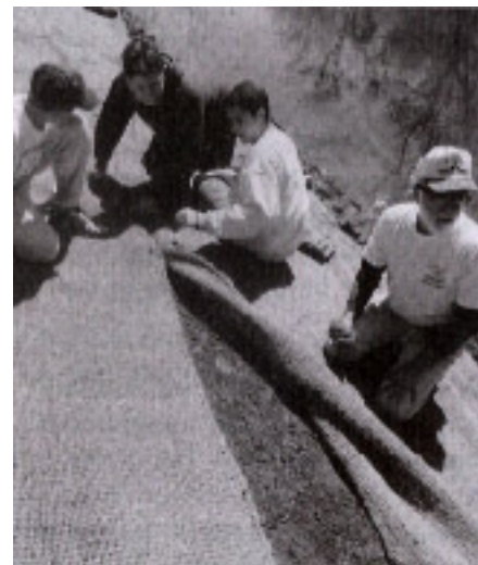
Volunteers install coconut coir matting on a recontoured streambank at Pennypack Creek in Fairmount Park, Philadelphia.
