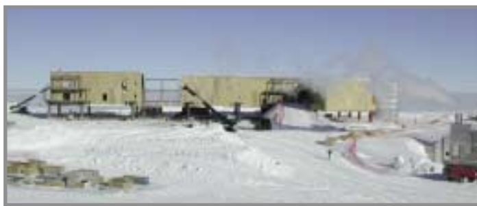
Photo by Jerry Marty/Special to The Antarctic Sun The new elevated station is now partially enclosed and work will continue through the winter.
