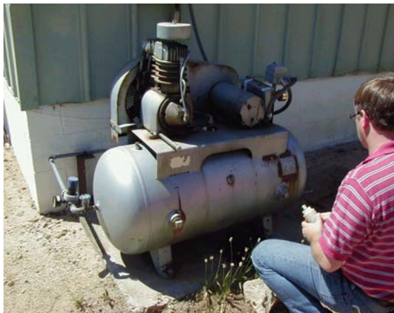
Air Receiver Tank
