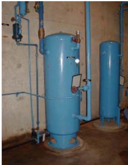
Air Receiver Tank
