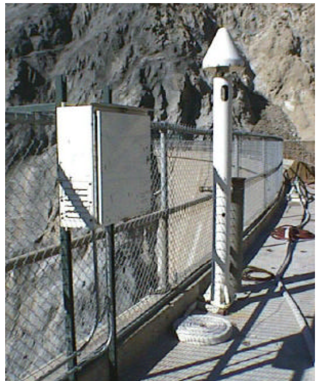
Figure 3. Station DAM2. The Dorne-Margolin choke ring antenna is mounted on a steel pier, and GPS receiver, modem and power supply are in the NEMA-type enclosure mounted to the fencing.
