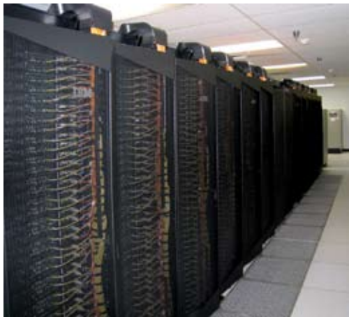
The NASA Center for Computational Sciences (NCCS) recently expanded its Discover supercomputer by integrating a 4,096-core IBM iDataPlex cluster, for a combined performance of 67 teraflops. NCCS plans to at least double the iDataPlex processor count during 2009. Jarrett Cohen, NASA Goddard
