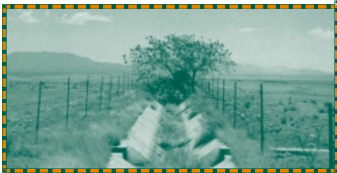
Water from the San Pedro River is diverted into cement-lined channels. Source: "Watershed at a Watershed," Arizona State University for Southwest Center for Environmental Research and Policy. Photo credit: Laurel McSherry.
