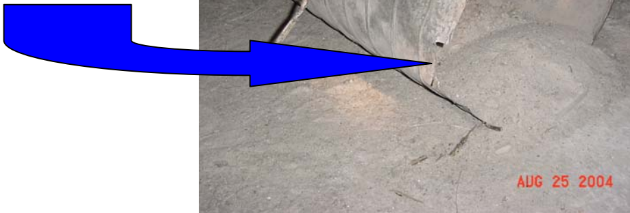
Figure 9: End of Vent Line 4
