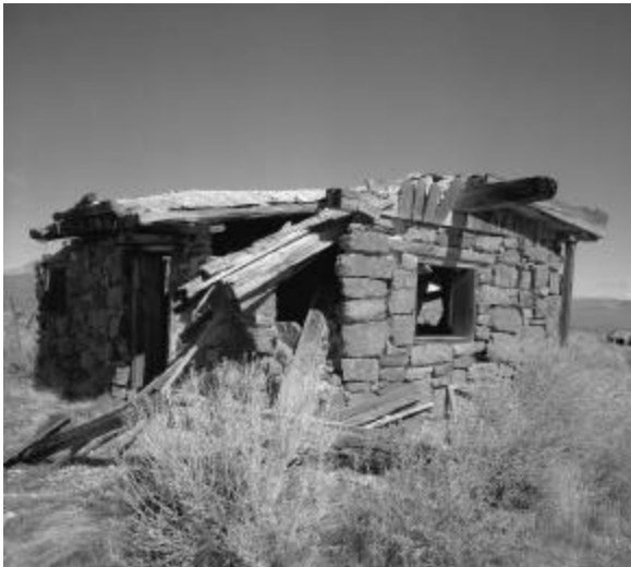
Ruins of herdsman's cabin at Tippetah Spring. Source: DOE, Nevada Operations Office.
