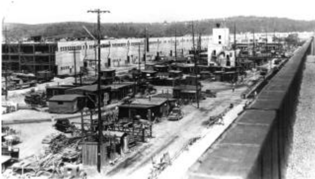
K-25 Gaseous Diffusion Plant under construction at Clinton. Source: Department of Energy.
