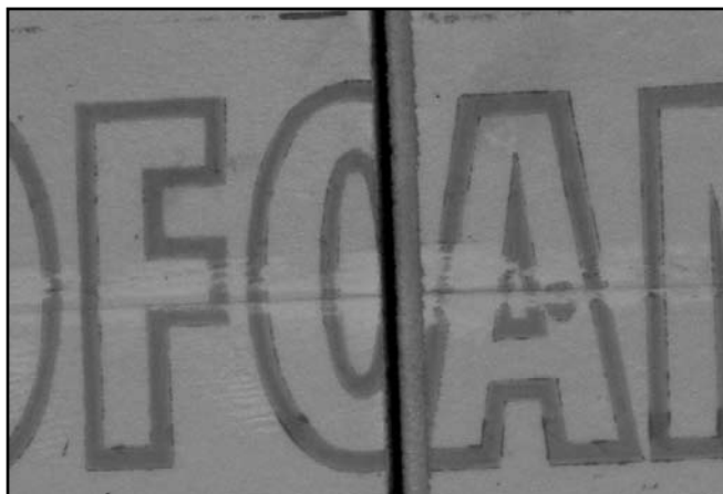
Figure 3. At some of the vertical foam joints, the tongues have separated entirely from the grooves.
