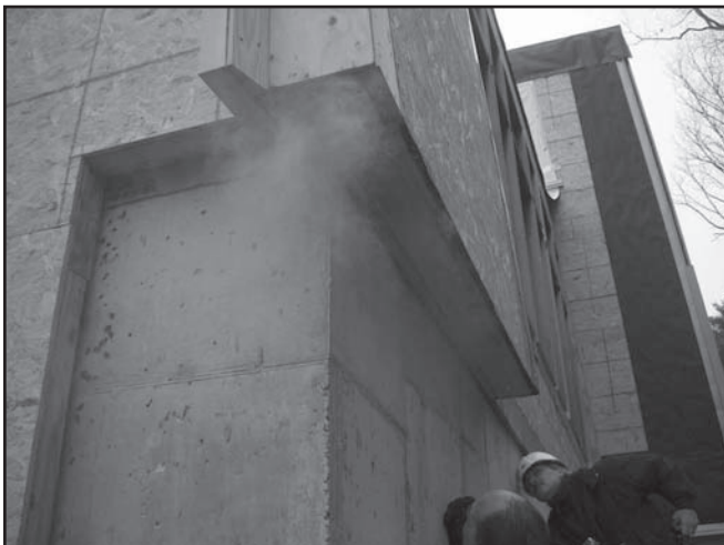
Figure 1. When theatrical fog is introduced into a pressurized building, it’s usually easy to spot any air leakage locations. [Photo credit: Dale Caldwell]
