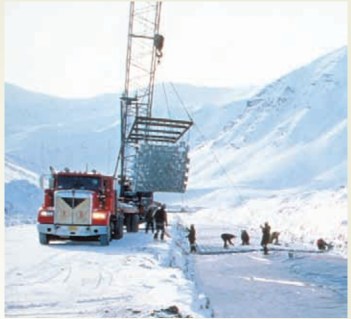
Pipeline workers endured temperatures to -50^{\circ}\text{F} or colder in winter, and mud, dust and clouds of mosquitoes in summer.
