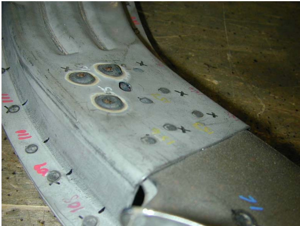
Photo 10. Standard MIG puddle welds were used where RSW guns would not fit into the box section.
