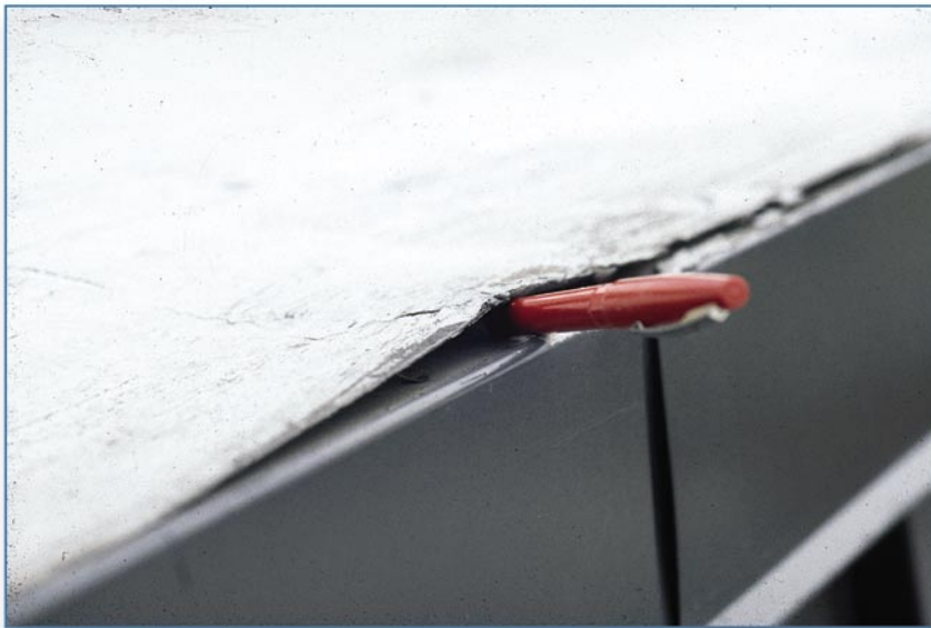
Figure 6-37 The metal edge flashing on this modified bitumen membrane roof was installed underneath the membrane, rather than on top of it and then stripped in. In this location, the edge flashing is unable to clamp the membrane down. At one area, the membrane was not sealed to the flashing (an ink pen was inserted into the opening prior to photographing). Wind can catch the opening and lift and peel the membrane.
