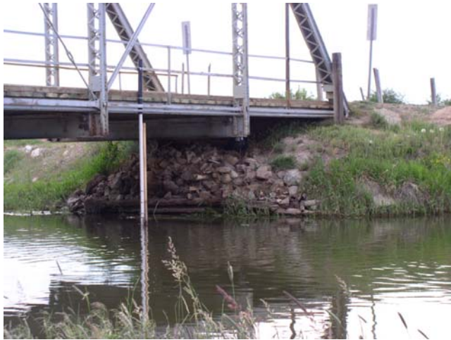
Figure 1 – Newly installed gaging station on the Bear River
