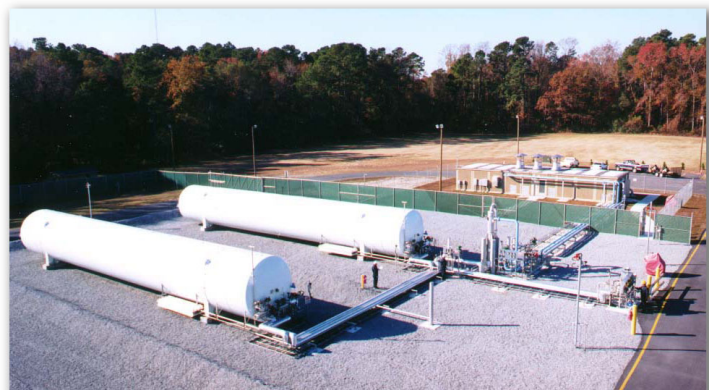
Typical LNG facility for baseload and peaking needs. – Photo Credit: Northstar Industries
