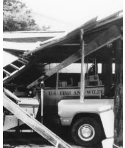
Storm damage. Besides damaging habitat used by several endangered and threatened species, last summer’s Hurricane Georges caused structural damage to Service facilities such as National Key Deer Refuge. Photo by Barry Stieglitz
