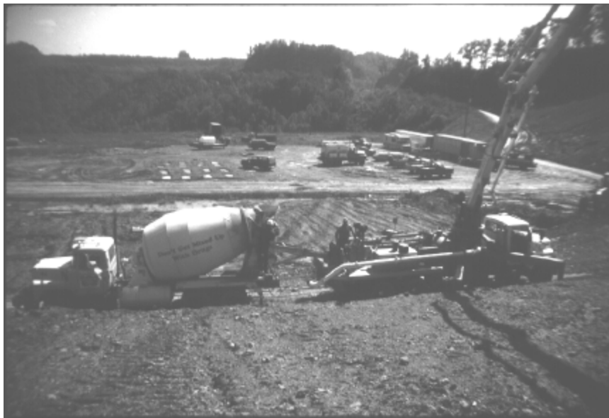
Figure 7. Photograph of field demonstration site, showing mixing truck (left) transferring grout to hopper in the piston pump (right).
