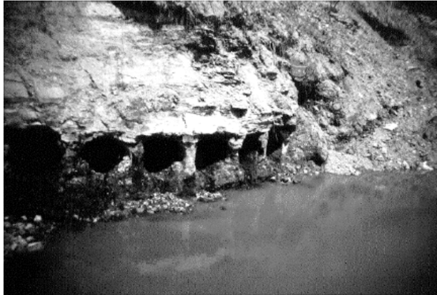
Figure 6. Abandoned highwall containing auger holes. Holes were initially plugged with rock and soil, and were exposed for this project. Each hole is approx. 3 ft. in diameter.
