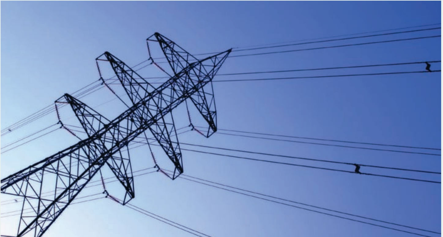
Transmission of new power can often be a challenge, but fortunately, a 138-kVA transmission line with plenty of spare capacity was available to U.S. Geothermal along the northern boundary of the Raft River geothermal field.
