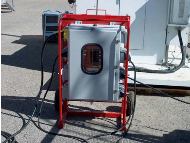
Figure 2-3. Electric distribution box used at DOE-NV.
