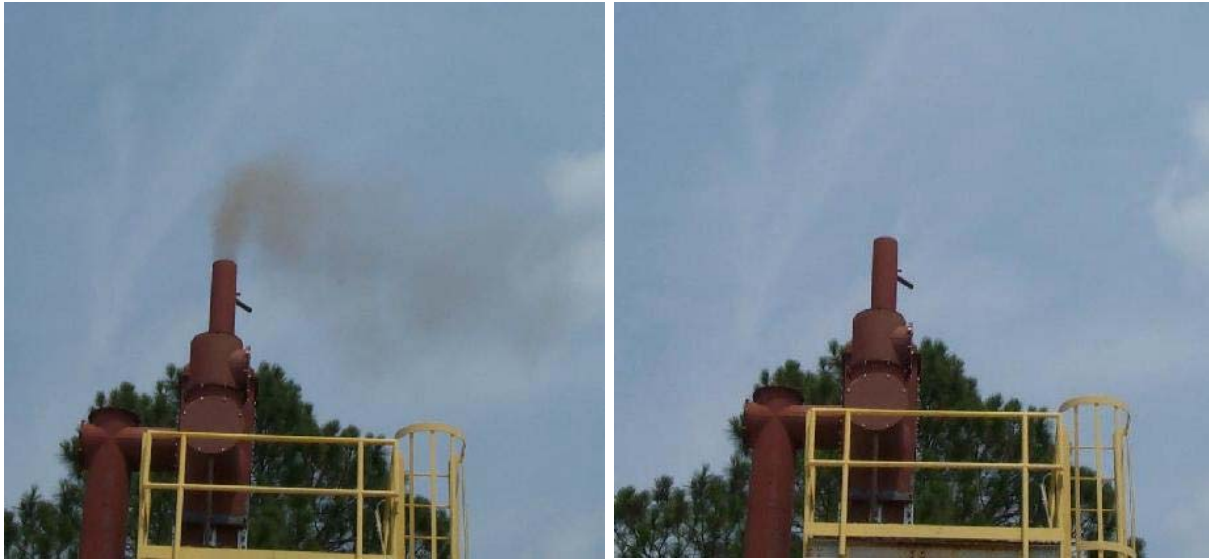
Figure 3. Dirty and clean stack (ten seconds after energizing field)
