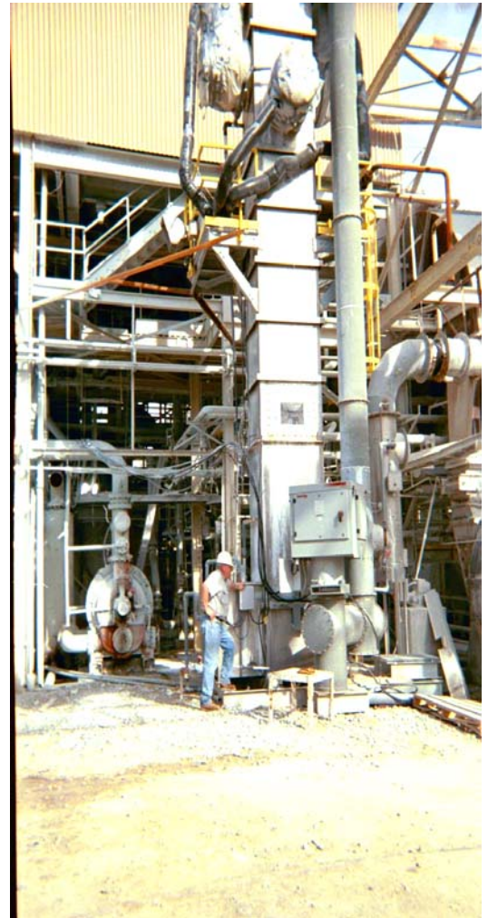
Membrane WESP Lime Kiln Pilot
