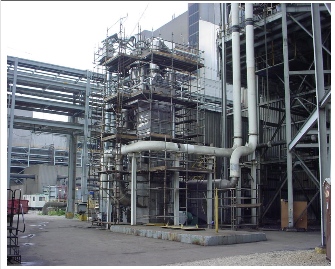
Pilot Metal tube (background) and Membrane Wet ESP (foreground) at First Energy's Bruce Mansfield, PA Plant.
