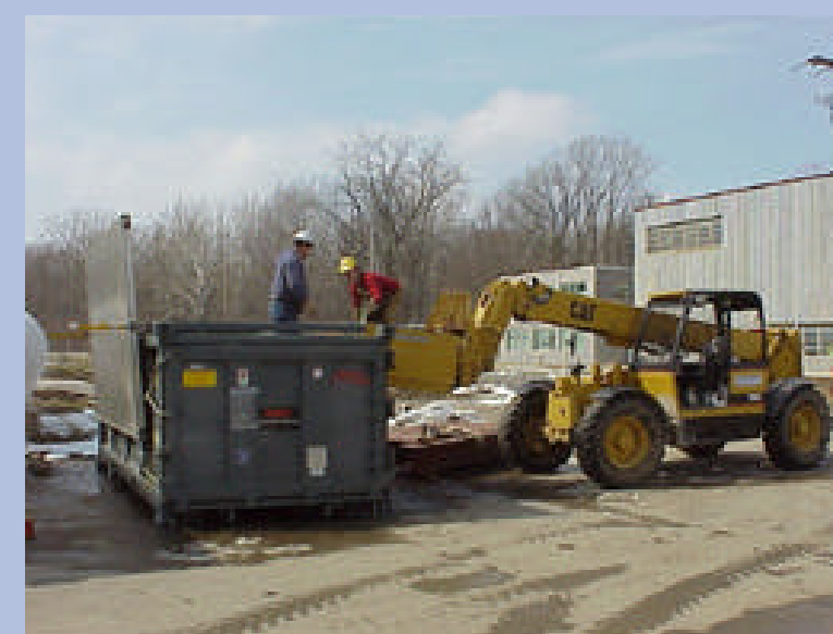
Then prepare to move the equipment into an Intermodal container - designed to ride atop both trucks and trains
