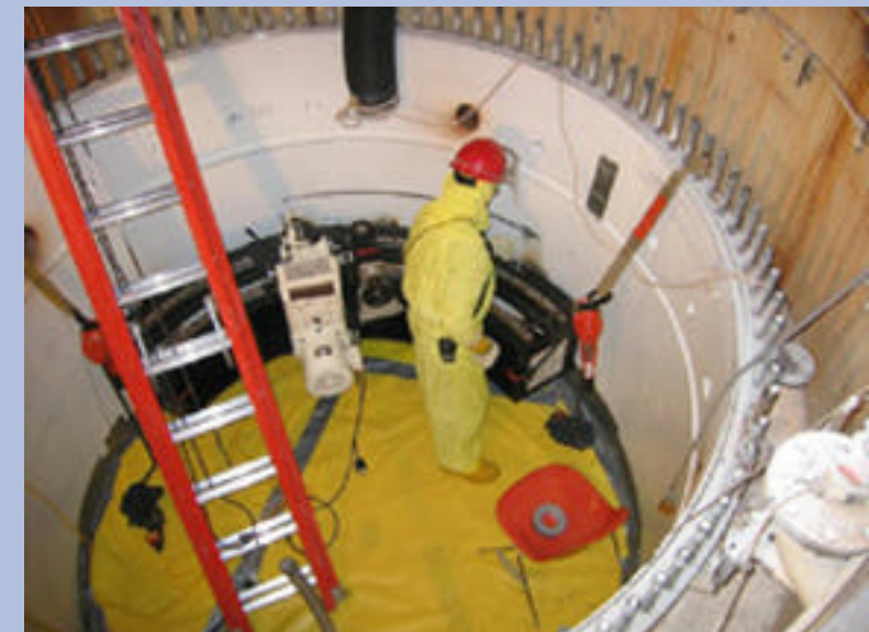
In July, workers began Phase 4 of segmentation, making the first cut on the reactor tank.
