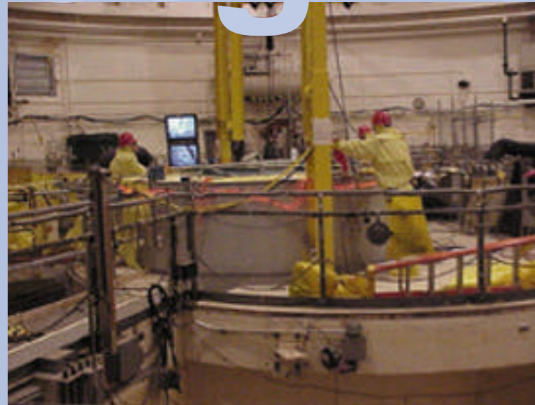
Workers used remotely operated tools and video cameras while removing the reactor internals.
