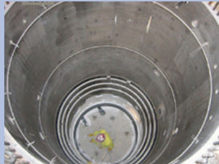
By June, workers had removed nearly all of the reactor internals. Standing inside the tank, a segmentation worker applies a compound to bind any loose contamination on the thermal shields, the last components they removed.
