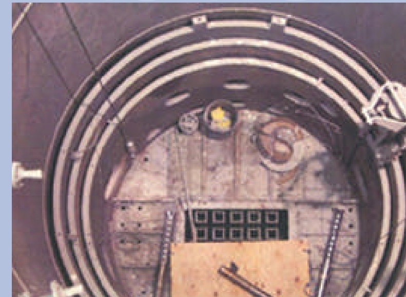
The project reached a major milestone in February, with the removal of the reactor core box.
