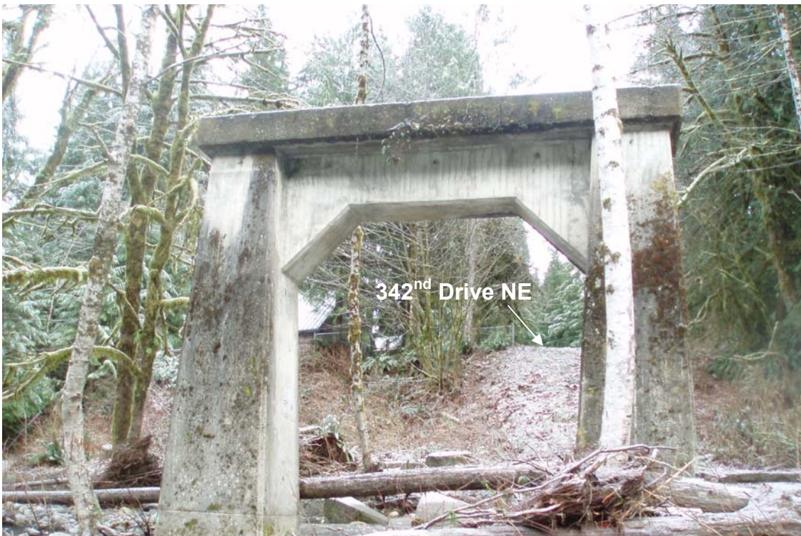
Existing concrete pier to be removed: Top photo is looking south. Bottom photo is looking north.
