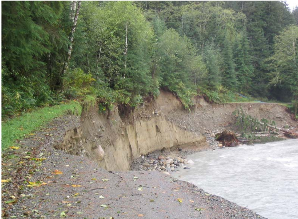
Site of Monte Cristo Grade Road washout, October 22, 2003 (looking downriver).
