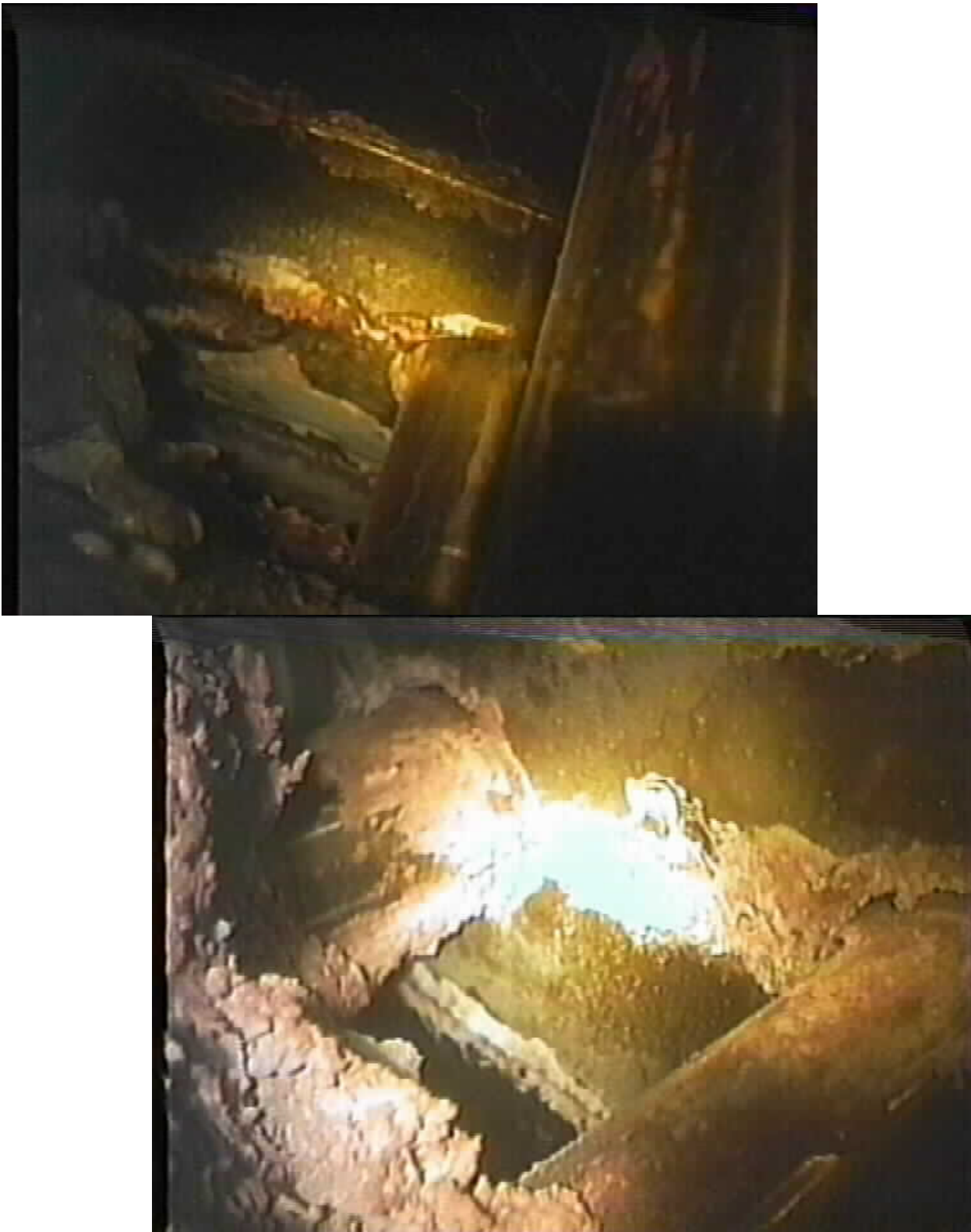
Figure 30. Flange Leakage Crusted On Side of Nozzles and Stalactites from Gaps in Insulation (8RFO)
