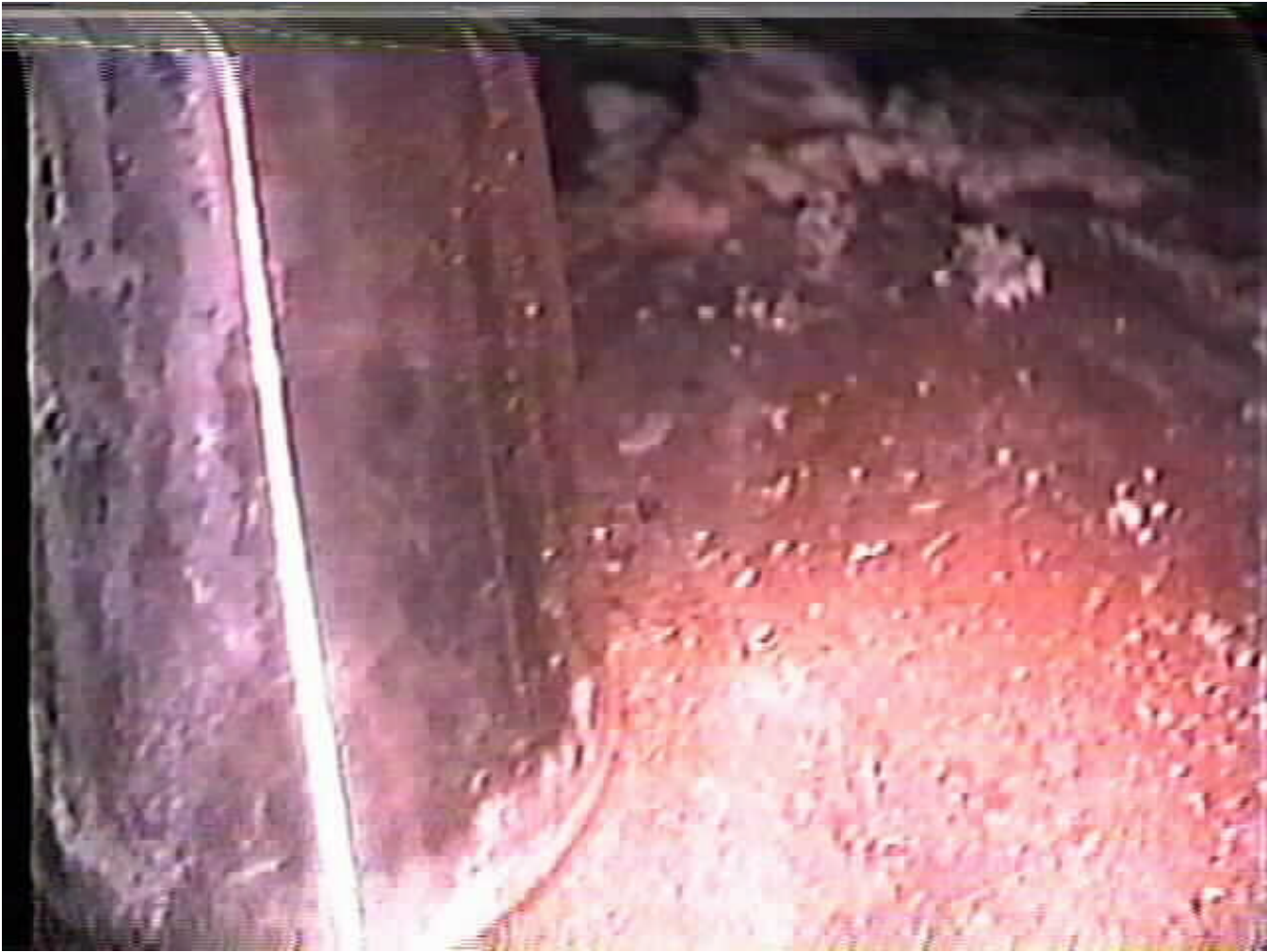
Figure 34. Boron Deposits Near Top of Reactor Vessel Head (10RFO)
