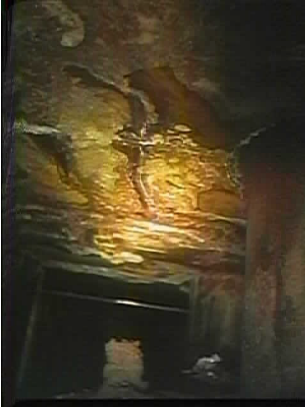
Figure 29. Flange Leakage with Stalactite Formation from Insulation and Stalagmite Formation on top of Reactor Vessel Head (8RFO)
