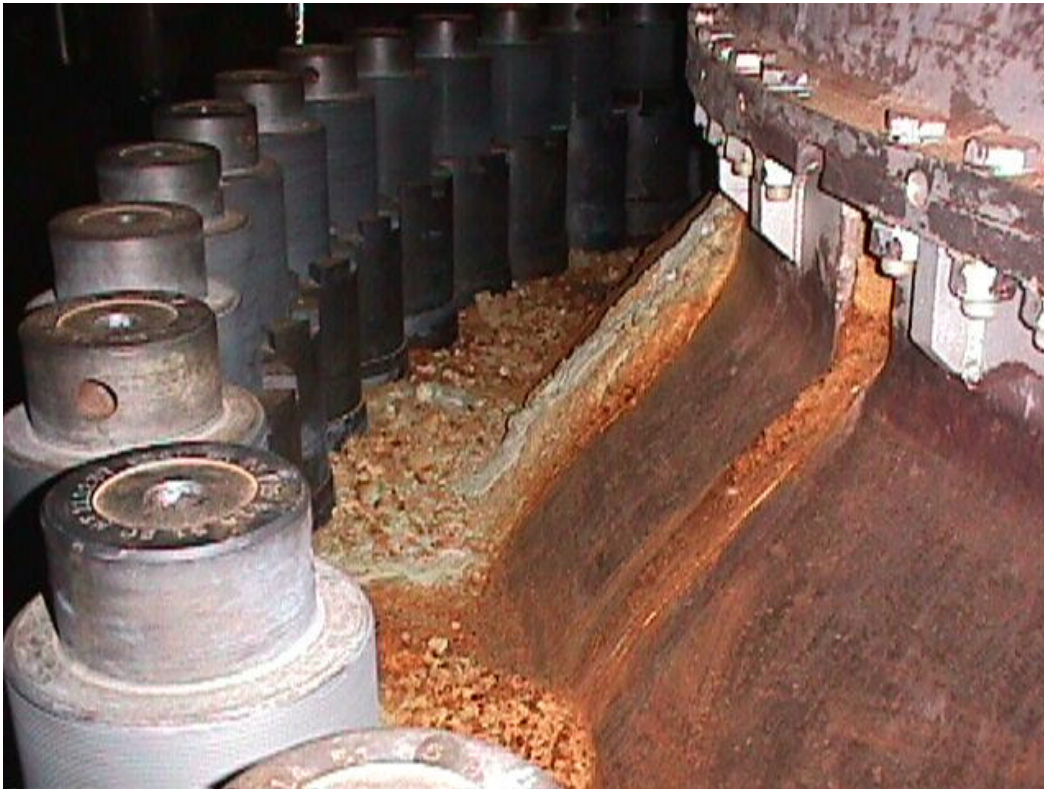
Figure 36. Red Rusty Boric Acid Deposits on Vessel Flange (12RFO)
