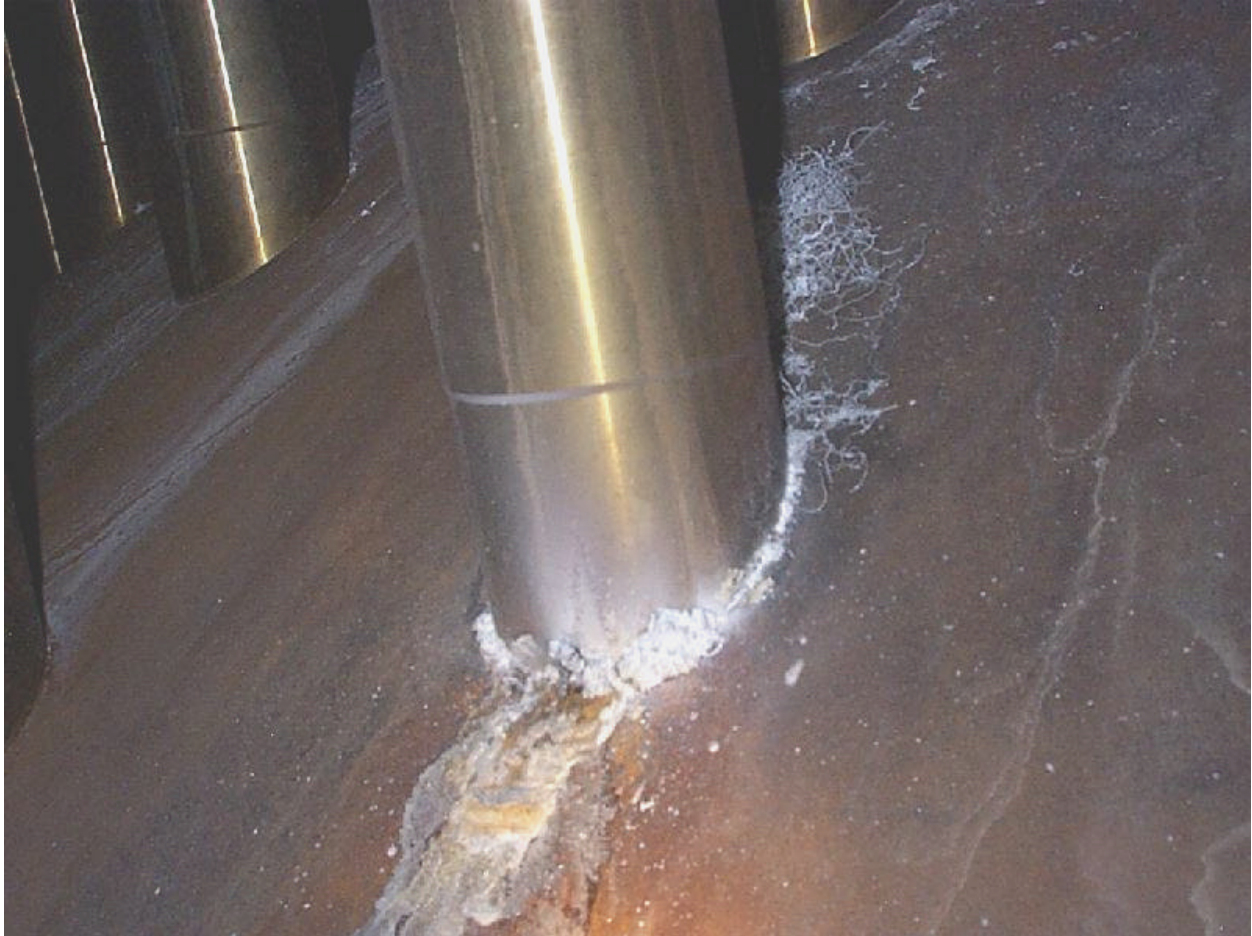
Figure 18. CRDM Nozzle Leakage Observed at Oconee 3
