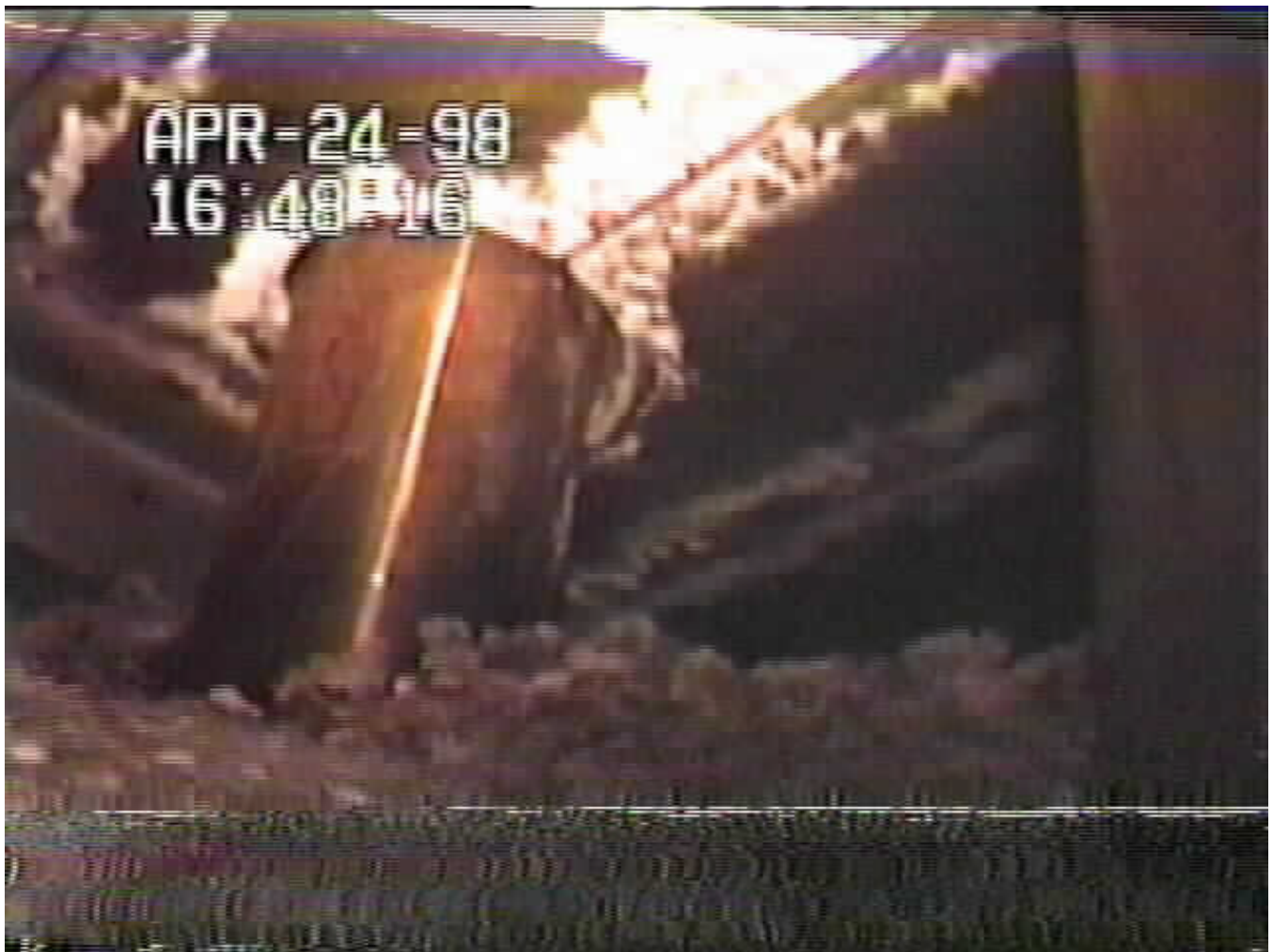
Figure 37. Boron Piled Under the Insulation (11RFO)
