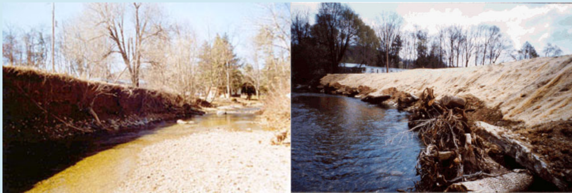
The streambank at the McDannel site was severely eroded at the beginning of the project in February 1999.
