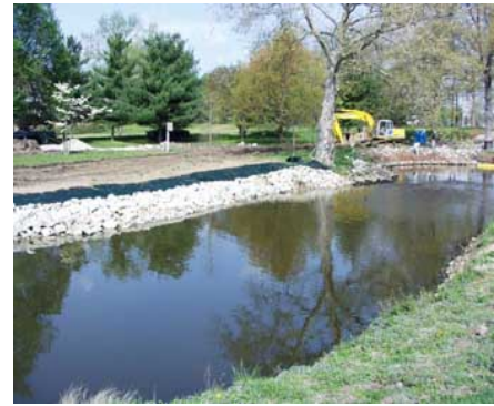
Figure 3.13 Riprap (Source: http://www.dnrec.state.de.us/dnrec2000/Divisions/Soil/dcmp/cdhydro.htm )
