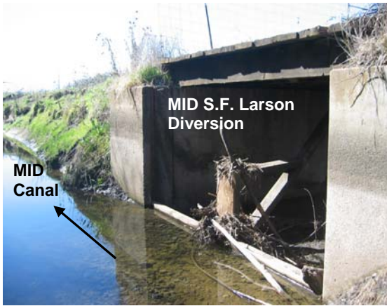
Figure 8. The MID diversion structure at South Fork Larson Creek during non-irrigation season.
