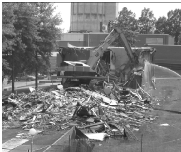
Buildings are coming down, too. Building 6003, one of three slated for demolition, was razed on June 25.
