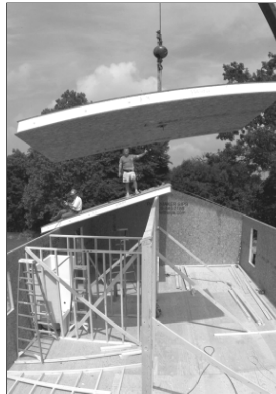
A roof panel is installed on the Lenoir City house, which went up in just three days. The house will have a heat-pump water heater and may be the testbed for a wood-fired microturbine that will generate electric power. The roof will also have solar panels.
