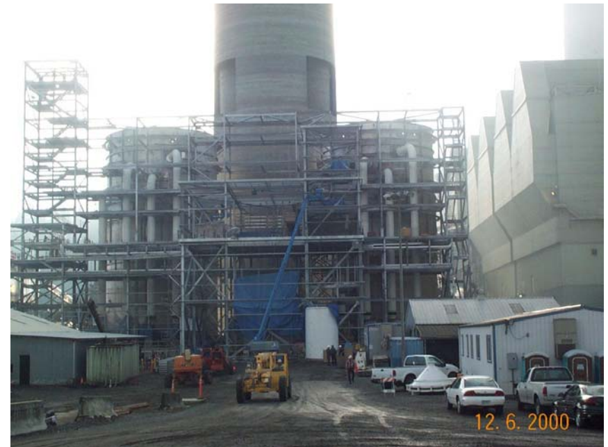
TransAlta Centralia Units 1 & 2 - 2 x 700 MW Lewis County, WA
