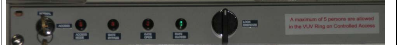
Figure 8: VUV Ring Access Control Panel
