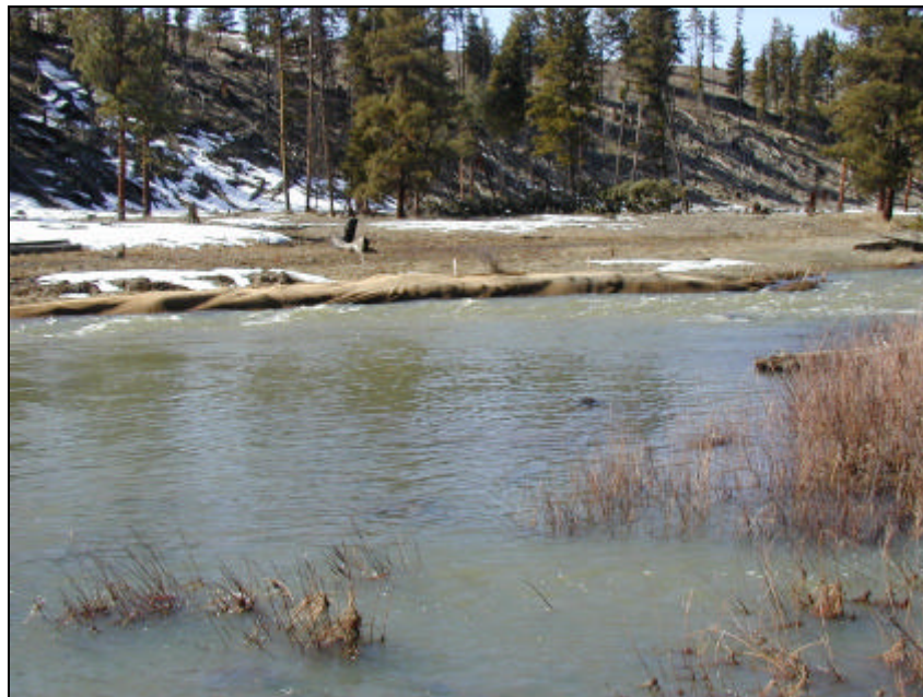
Meadow Creek stream channel meander construction. Photo illustrates bioengineering technique involving use of coconut fabric.
