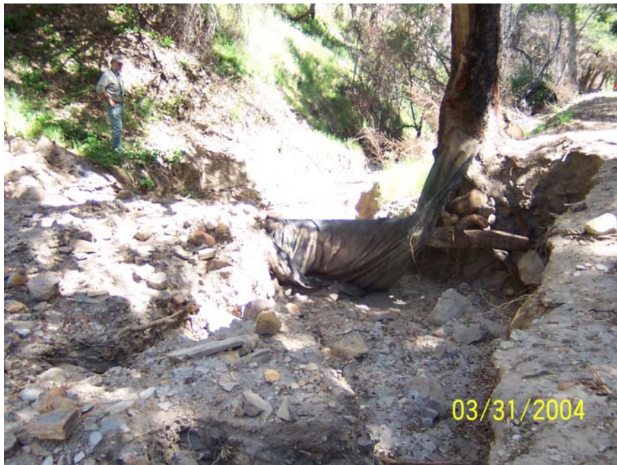
Figure 29 - Failed log-barrier checks dams in Dominguez Canyon, southern California.
