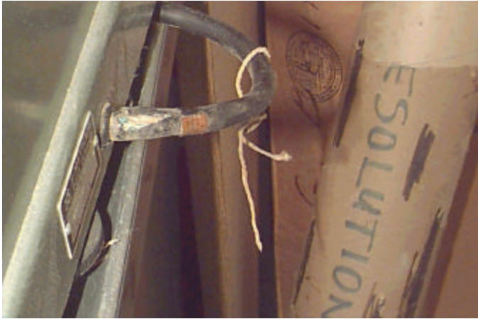
Figure 4. Poor maintenance of equipment: frayed power cord.
