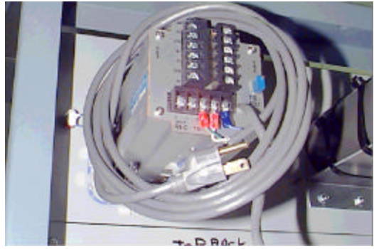
Figure 1. Power circuit and exposure to potentially energized terminals.
