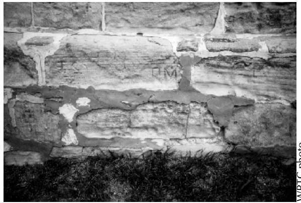
Figure 19. The use of hard portland cement mortar and sloppy pointing technique have aided in the deterioration of this soft sandstone wall.
