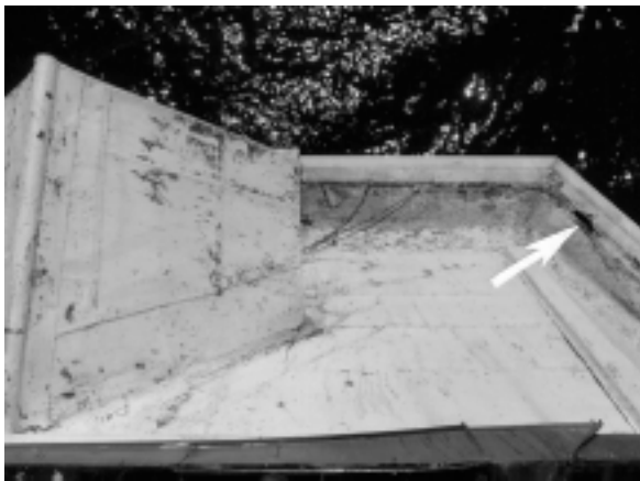
Figure 9. View of built-in gutter system on a mansard-style roof; the arrow indicates where a fist-size hole exists. This hole allows water to enter the interior of the lighthouse.
