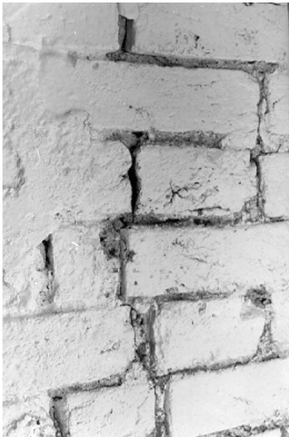
Figure 21. Detail of eroded pointing.
