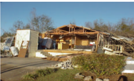
F2 tornado damage in Coldwater (Calhoun County) on 11/24/ 2004.
