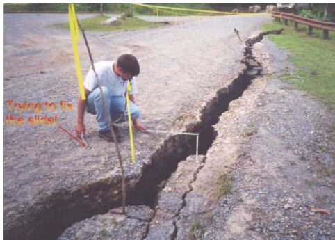
Figure 2. Initial Landslide crack developed through the roadway embankment
